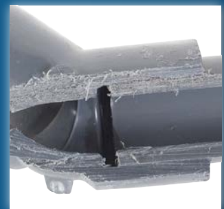
PVC Joint close-up of gap that can be created at joints, allowing for build up of biofilm.
